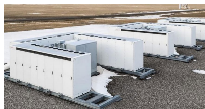
Battery Energy Storage System (BESS)
